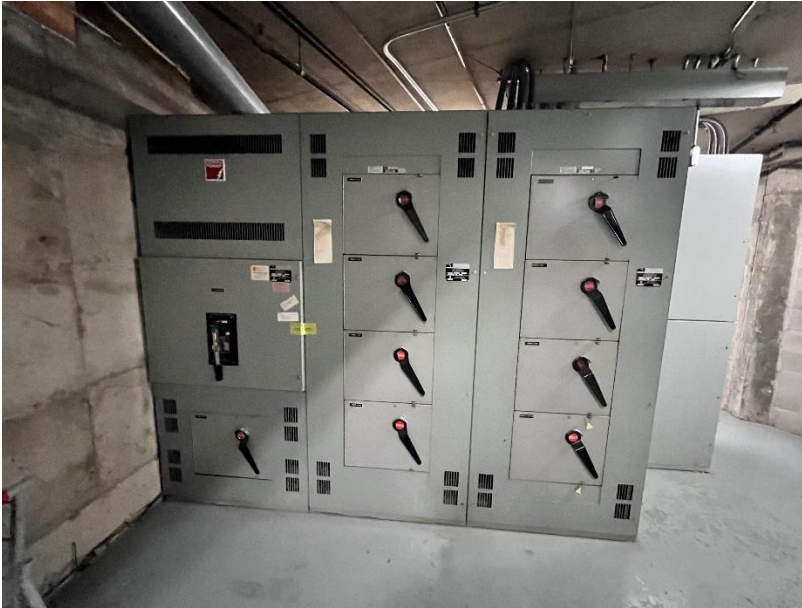
Figure 3 Panneau de distribution principal
